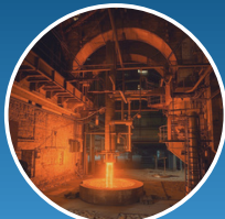
Induction melting furnaces
